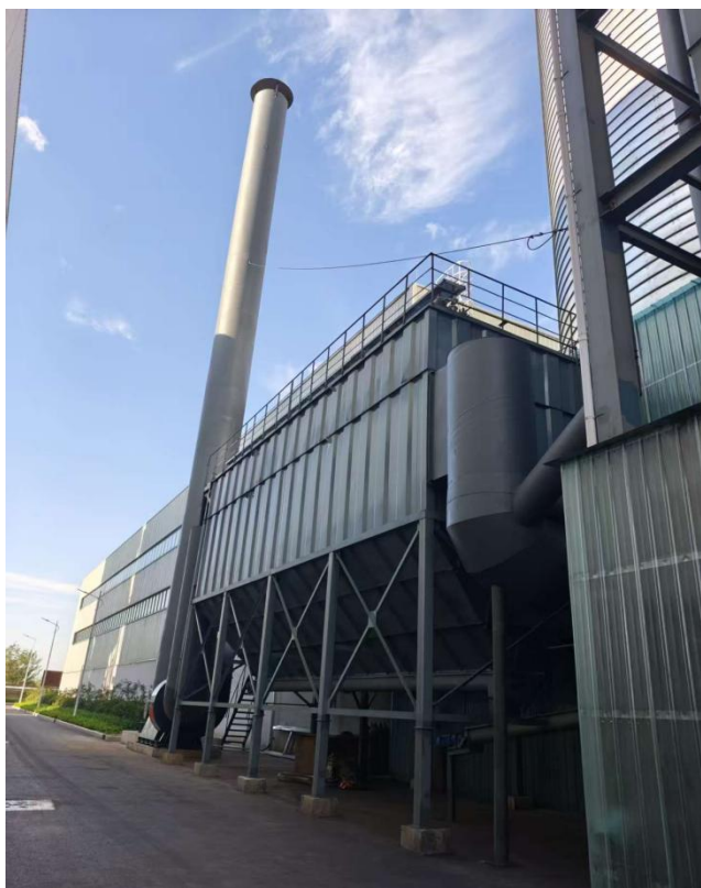
TA001 脉冲除尘器+35mDA001 排气筒
